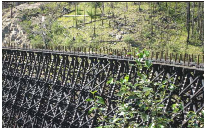
Trestle No. 4 nearing completion in the Myra Canyon. Photographs courtesy of Katim Enterprises Ltd.
