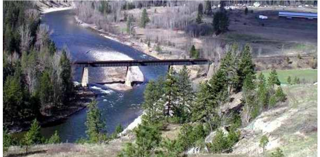
Canadian Pacific Railway's St. Mary's River Bridge to be soon converted to a trail bridge. Al Skucas photo.
