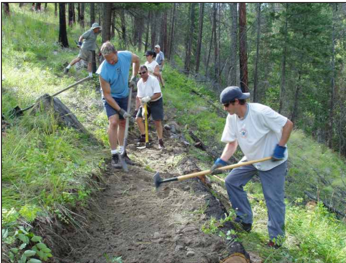
July 2007: FOSS volunteers build a section of trail through Kelowna's Priest Creek Linear Park (the trail provides public access to Myra-Bellevue Provincial Park).
